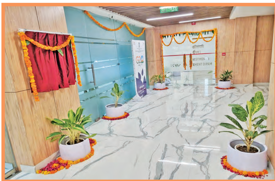
Interior/ Renovations work at Department of Investment and Public Asset Management, New Delhi
