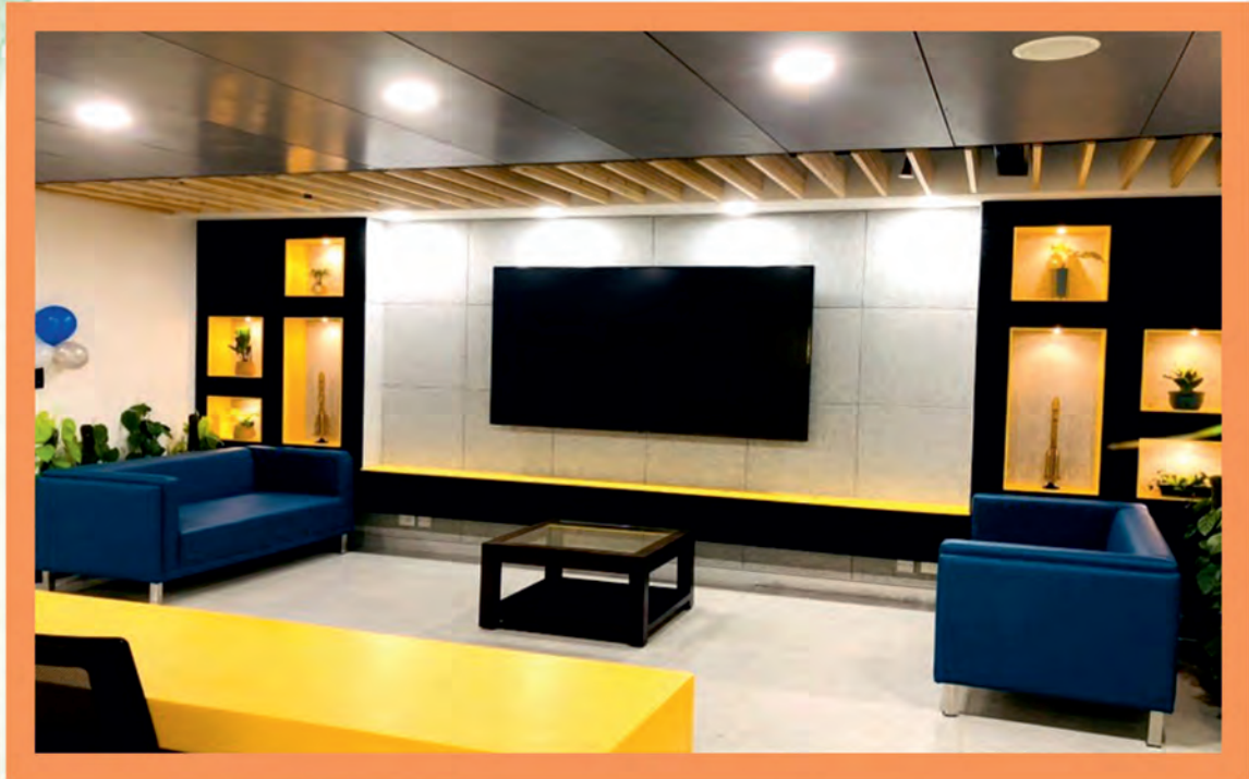
Interior Fit out work at Hindustan Aeronautics Limited, East Kidwai Nagar, New Delhi
