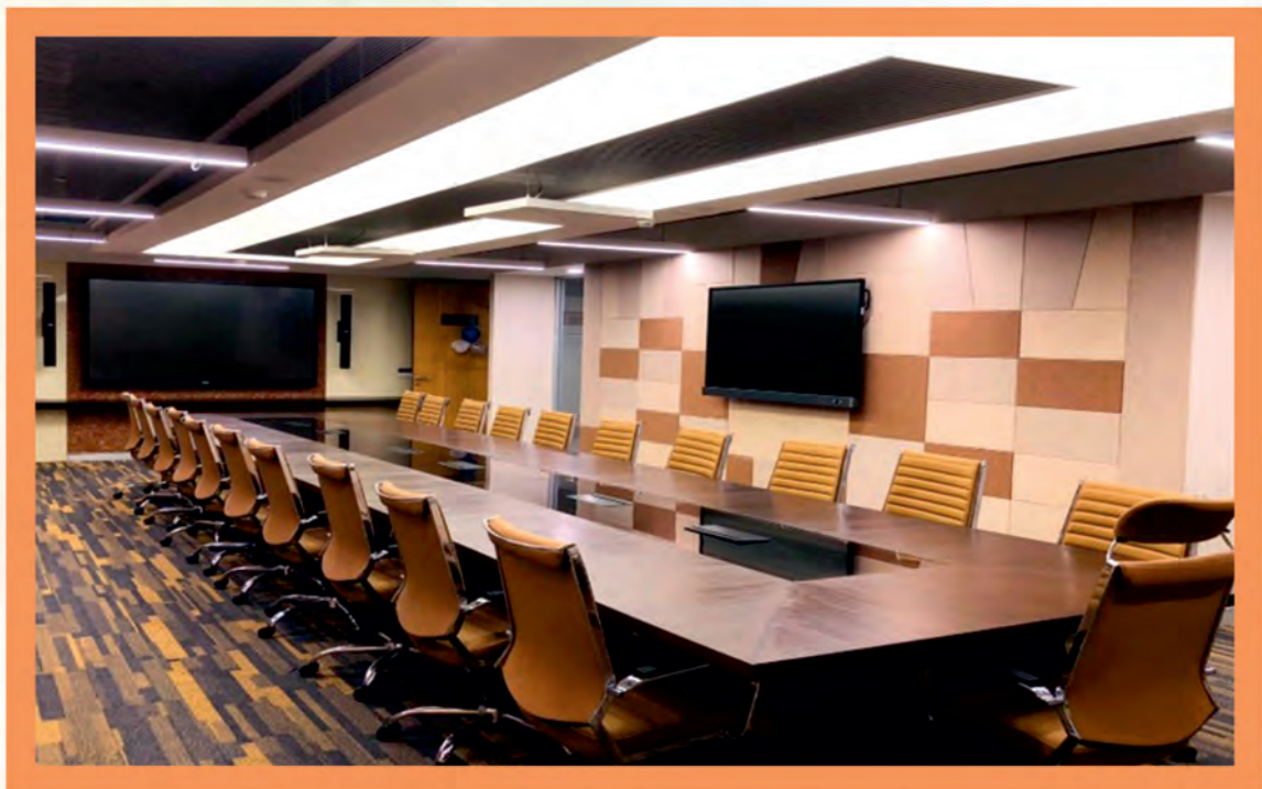
Interior Fit out work at Hindustan Aeronautics Limited, East Kidwai Nagar, New Delhi
